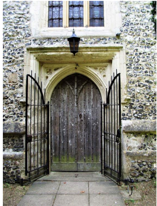
This photograph was taken on the 22 nd of July 2009 and shows the C15th west door and its contemporary ornamental limestone surround
